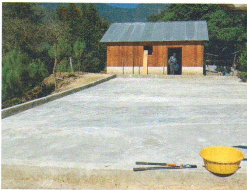
Cement slab for drying coffee beans
